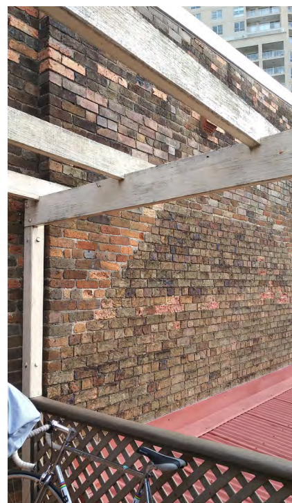
Figure 157: View of brick repairs to external wall of SBW Stables Theatre. Roof over kitchen visible.
