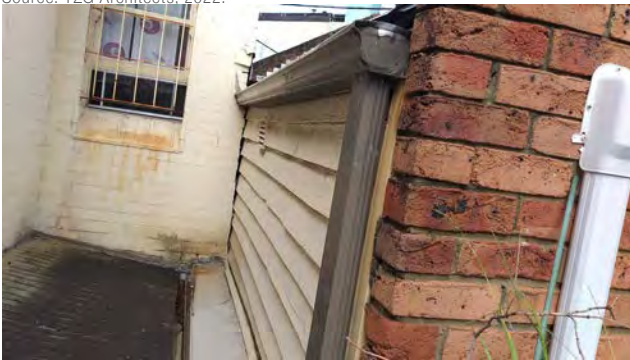
Figure 96: View of junction with neighbouring terrace house and timber weatherboard cladding on south facade at 12 Nimrod Street from upper level terrace.
