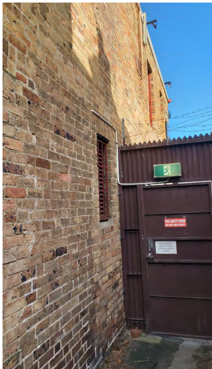
Figure 103: Evidence of repointing and brick repairs to facade of theatre in rear lane.
